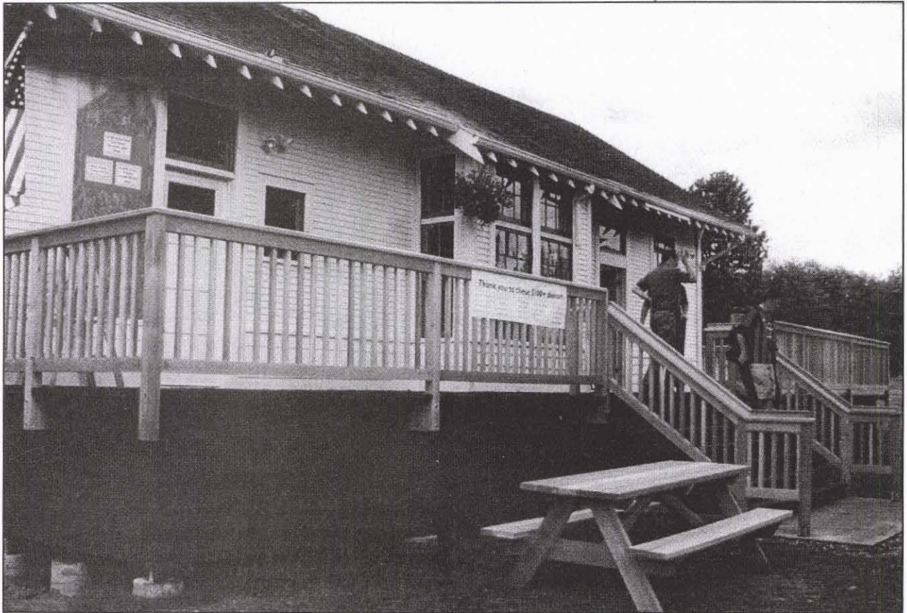
Steps, deck and picnic tables built by Carl Seip and his volunteers for access to the historic Chicago, Milwaukee, St. Paul, and Pacific Railroad depot at Depot Park, Duvall
